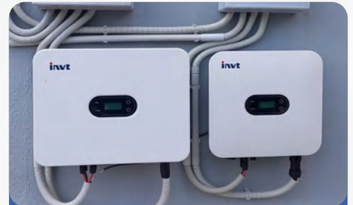
16kW Solar System in Greece (XG6KTL、XG10KTR)
