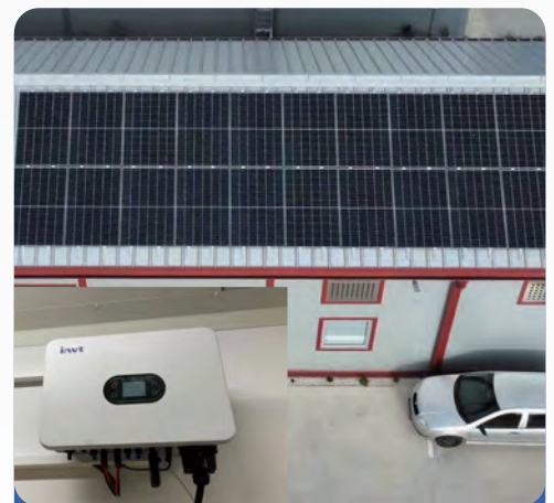
25kW Solar System in Slovakia (XG25KTR)
