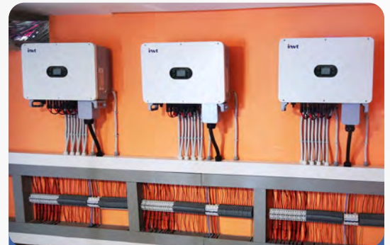
180kW Rooftop PV Plant in Lebanon (XG60KTR)
