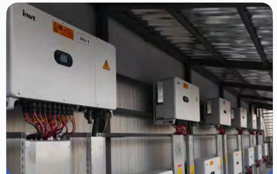
2MW Rooftop PV Plant in Türkiye (XG110KTR)
