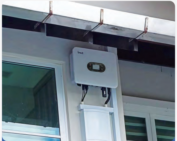
12kW Solar System in Malaysia (XG12KTR)
