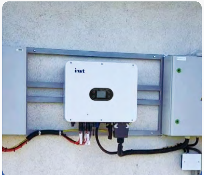
30kW Solar System in Serbia (XG30KTR)
