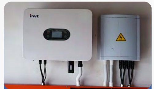
25kW Solar System in Malaysia (XG25KTR)
