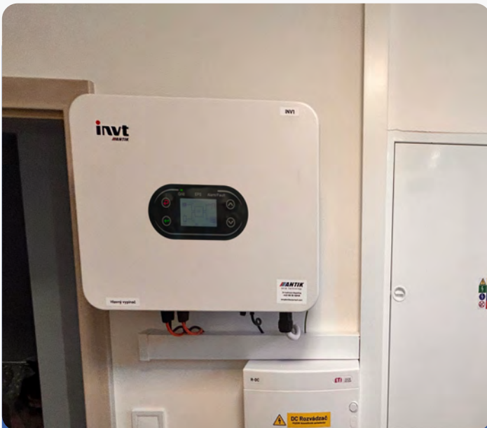
10kW Solar System in Slovakia (XG10KTR)
