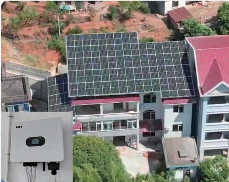
40kW Solar System in Jiangxi, China (XG40KTR)
